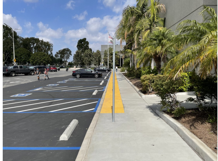
Swing Space—Hotel, Restaurant, and Culinary Arts: Americans with Disabilities Act (ADA) Parking Lot 1— Completed Construction
